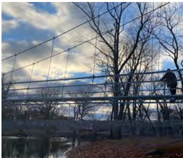
Steven Choate, walking across the bridge - which doesn't have a deck!
