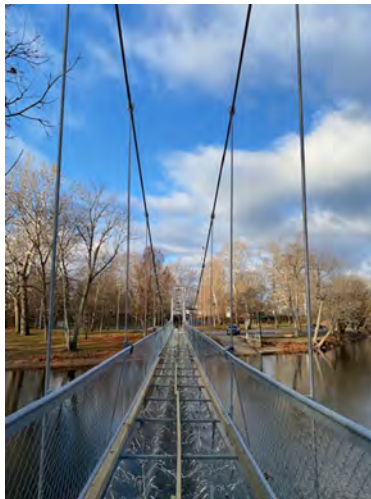
No deck... work has been halted for a while by the Town. But the morning is becoming brighter!
