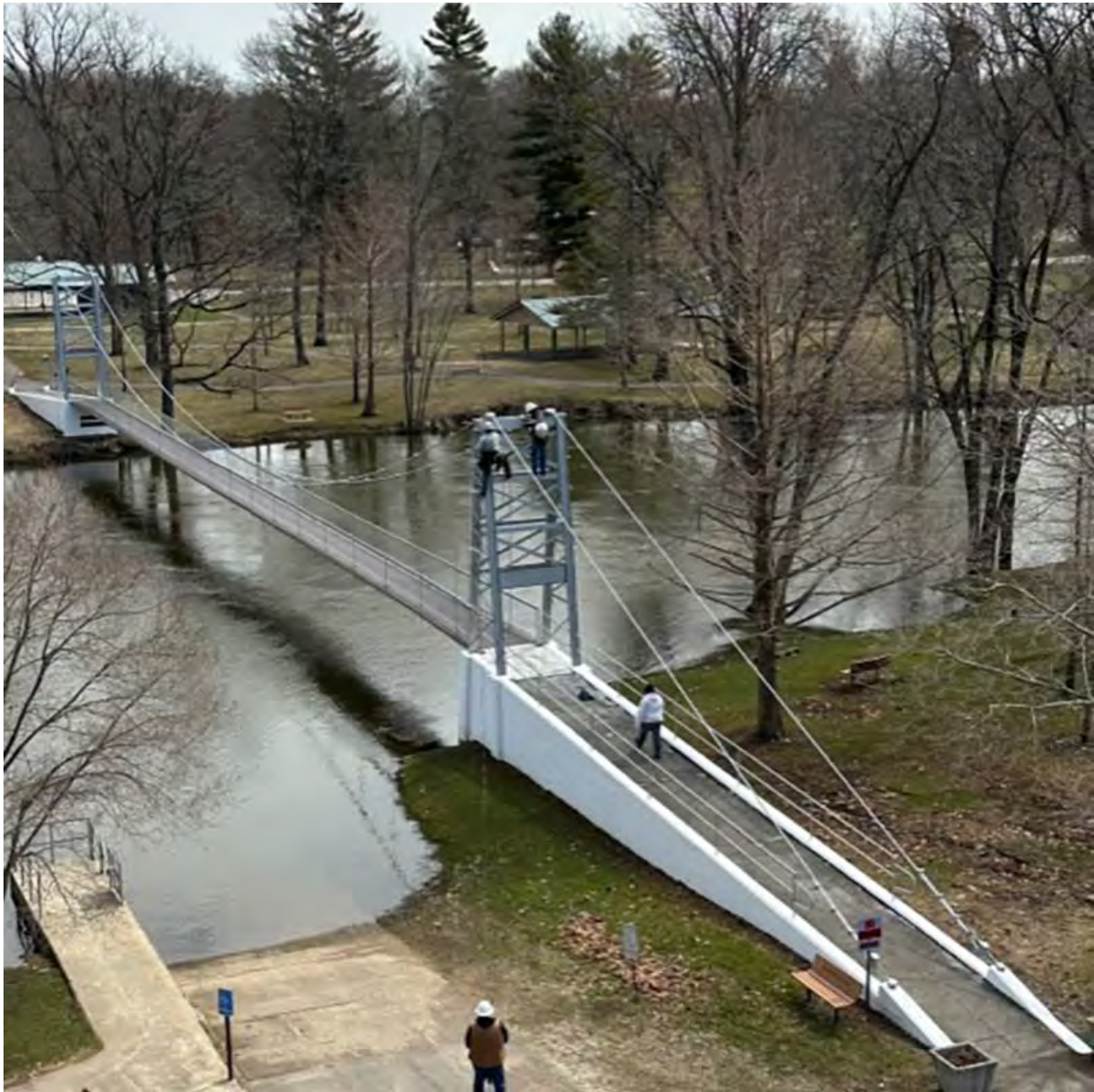
The bridge is open to pedestrian traffic!!!! Work still continues in this photo.
